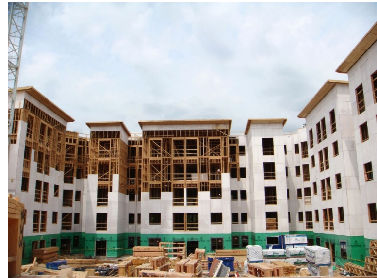
Exterior walls, Type III Construction The Varsity, University of Maryland, College Park, MD
